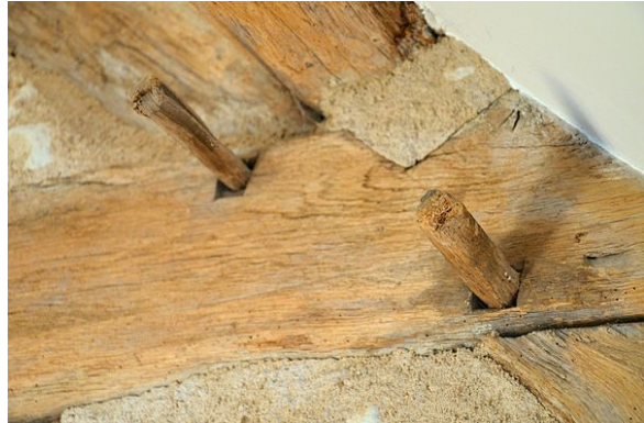
Joints in an ancient French roof, the wooden pegs hold the mortise and tenon joinery together.
