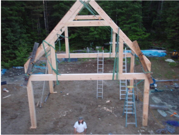
This is a part of a timber frame, before pegs are inserted
