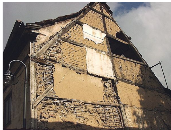
Half-timbered wall with three kinds of infill, wattle and daub, brick, and stone. The plaster coating which originally covered the infill and timbers is mostly gone. This building is in the central German city of Bad Langensalza.
