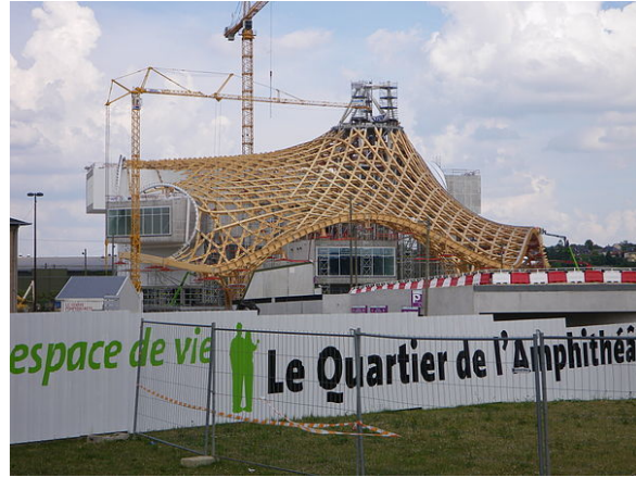
The Centre Pompidou-Metz museum under construction in Metz, France in 2009. The building possesses one of the most complex examples of carpentry built to date and is composed of 16 kilometers of glued laminated timber for a surface area of 8,000 m 2 .
